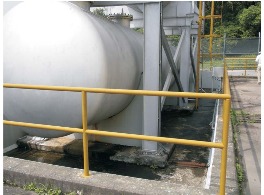
Above ground storage tanks
