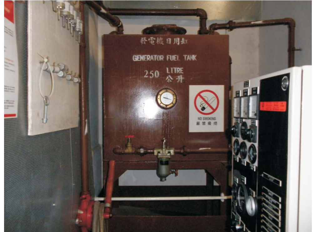
Above ground oil storage tank
